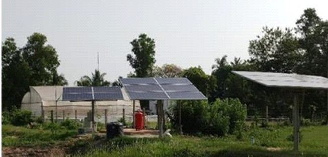
Figure 3: Installed solar PV Pumping System at IIT Kharagpur
